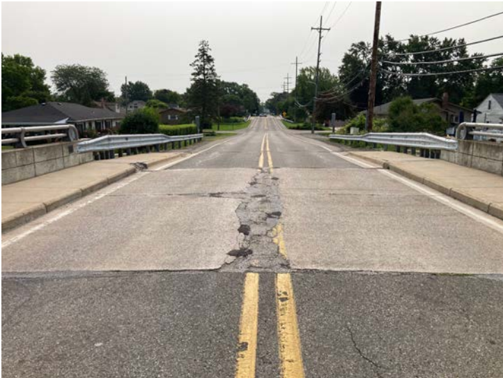
Document Name: IMG_4531.JPG Category: Approach Span Number: Comments: Looking east through structure
