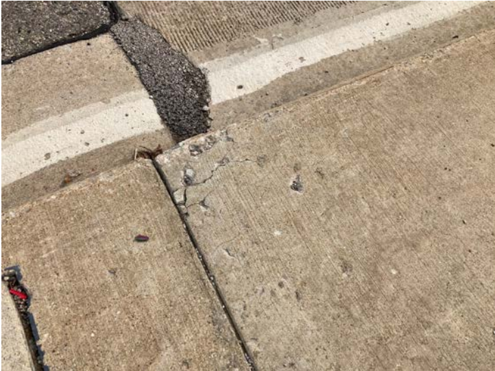
Document Name: IMG_4543.JPG Category: Deck Span Number: Comments: Incipient spall, SW sidewalk corner
