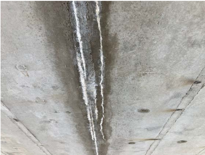
Document Name: IMG_4548.JPG Category: Superstructure Span Number: Comments: Leaching crack, beam 7s
