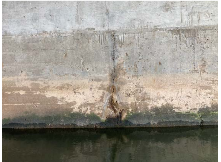
Document Name: IMG_4549.JPG Category: Substructure Span Number: Comments: Vertical crack in abutment, typical
