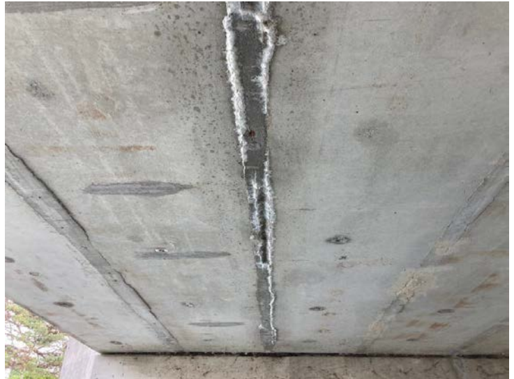
Document Name: IMG_4568.JPG Category: Superstructure Span Number: Comments: Leakage between beams
