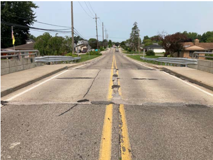
Document Name: IMG_4552.JPG Category: Approach Span Number: Comments: Looking west through structure
