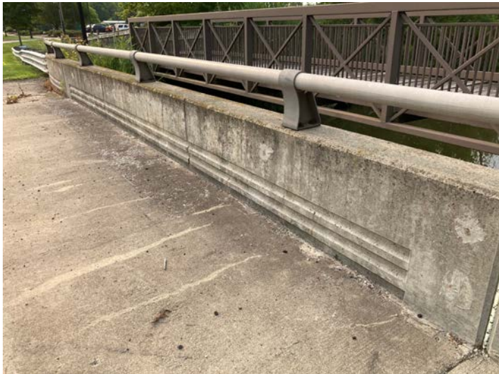
Document Name: IMG_4497.JPG Category: Railing Span Number: Comments: South rail
