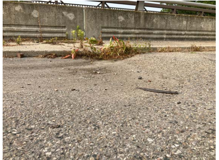
Document Name: IMG_4499.JPG Category: Approach Span Number: Comments: Settlement at approaches
