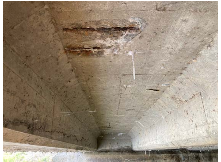
Document Name: IMG_4507.JPG Category: Deck Span Number: Comments: Deck bottom
