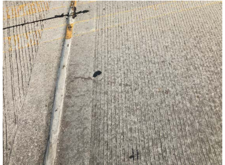
Document Name: IMG_4523.JPG Category: Deck Span Number: Comments: Longitudinal cracks in deck surface
