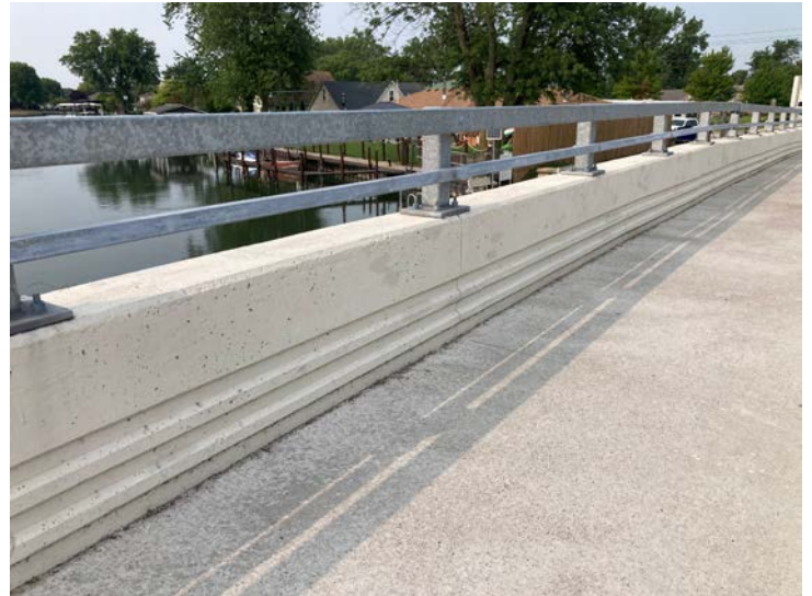
Document Name: IMG_4518.JPG Category: Railing Span Number: Comments: South rail
