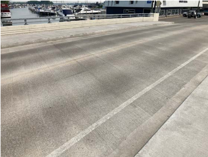
Document Name: IMG_4514.JPG Category: Deck Span Number: Comments: Deck surface
