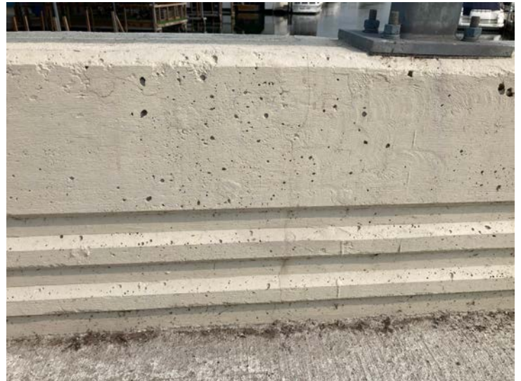
Document Name: IMG_4524.JPG Category: Railing Span Number: Comments: HL vertical crack in north rail
