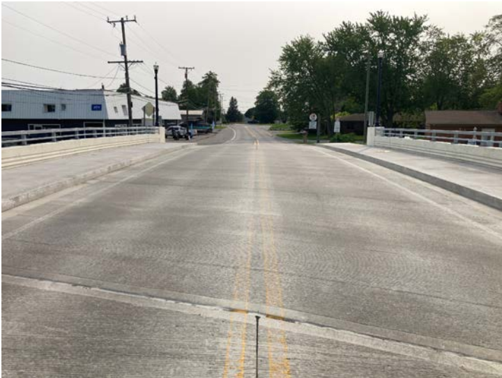
Document Name: IMG_4511.JPG Category: Approach Span Number: Comments: Looking east through structure
