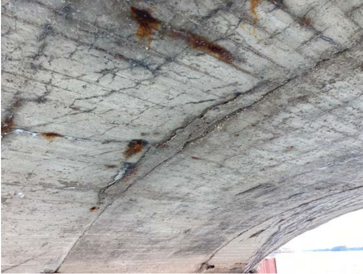
Document Name: IMG_4589.JPG Category: Superstructure Span Number: Comments: Incipient spall along construction joint
