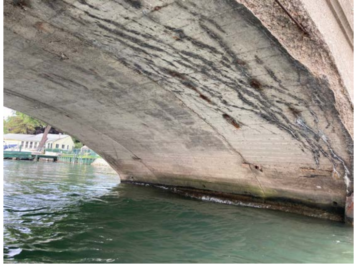
Document Name: IMG_4586.JPG Category: Superstructure Span Number: Comments: West half of arch
