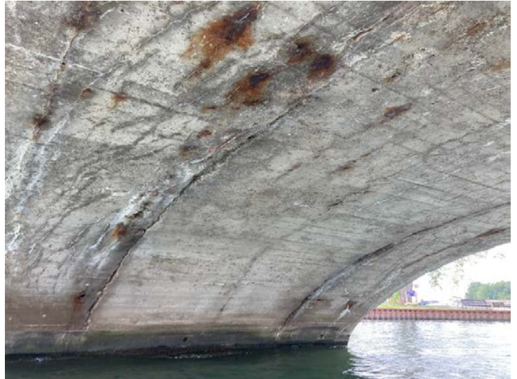
Document Name: IMG_4588.JPG Category: Superstructure Span Number: Comments: East half of arch
