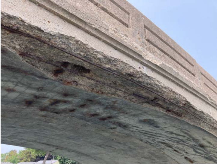
Document Name: IMG_4584.JPG Category: Superstructure Span Number: Comments: Spall to steel with 2 debonded bars along north fascia.
