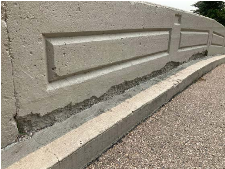
Document Name: IMG_4582.JPG Category: Railing Span Number: Comments: Spalling in rails
