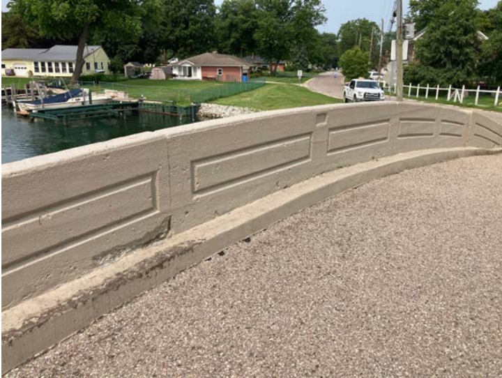
Document Name: IMG_4578.JPG Category: Railing Span Number: Comments: South rail
