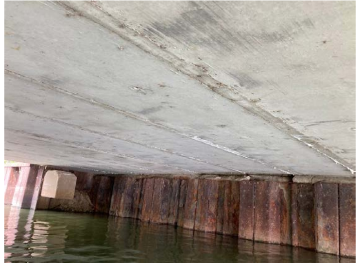
Document Name: IMG_4609.JPG Category: Superstructure Span Number: Comments: Leakage at beams
