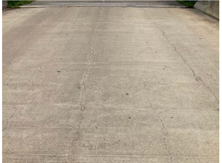
Document Name: IMG_4605.JPG Category: Deck Span Number: Comments: Longitudinal cracks in deck surface
