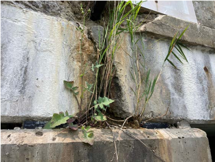
Document Name: IMG_4612.JPG Category: Superstructure Span Number: Comments: Spall to steel in beam 10s
