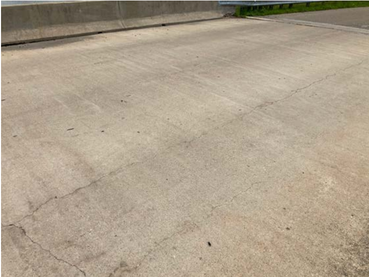
Document Name: IMG_4598.JPG Category: Deck Span Number: Comments: Deck surface, span 2w
