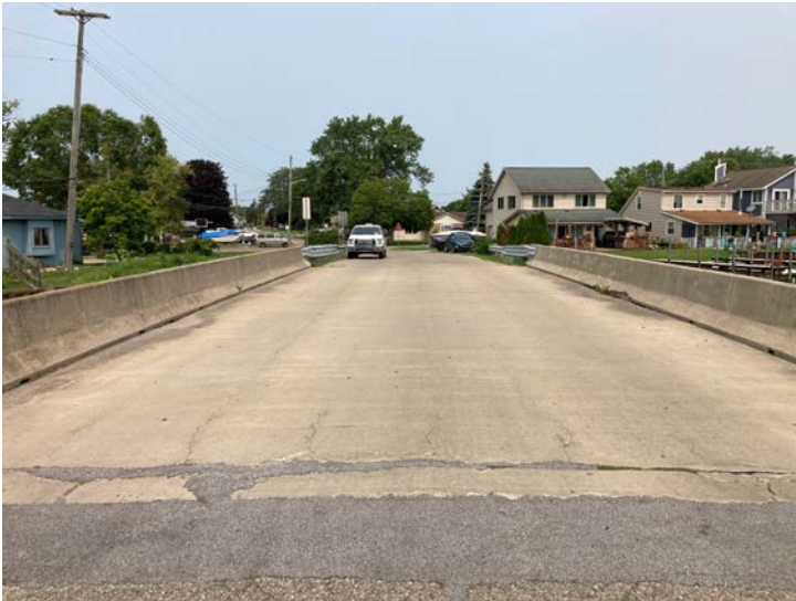
Document Name: IMG_4593.JPG Category: Approach Span Number: Comments: Looking west through structure
