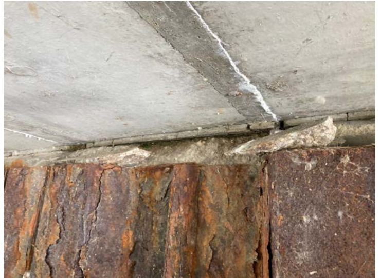
Document Name: IMG_4611.JPG Category: Substructure Span Number: Comments: Spalling of concrete at top of abutments
